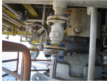
Figure 6 Upstream Pipeline Sensor
